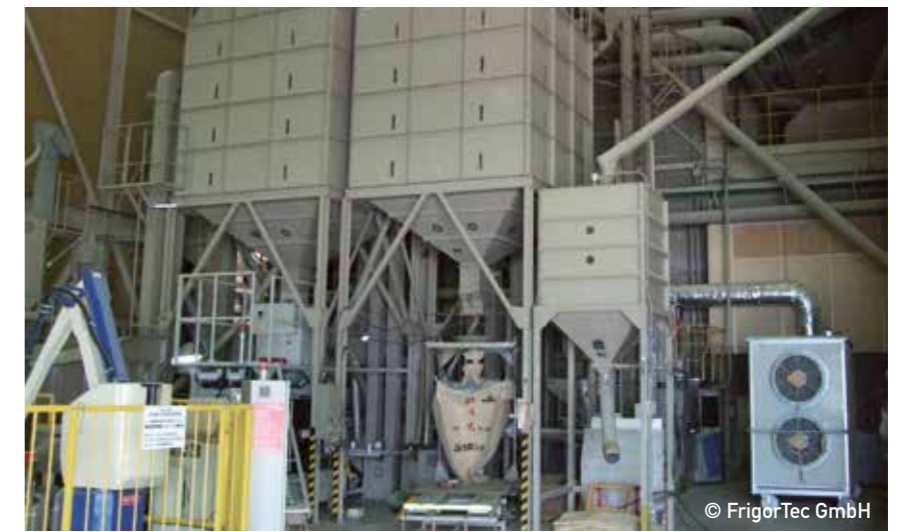
13 White rice silo with GRANIFRIGOR™ cooling unit in a rice mill
