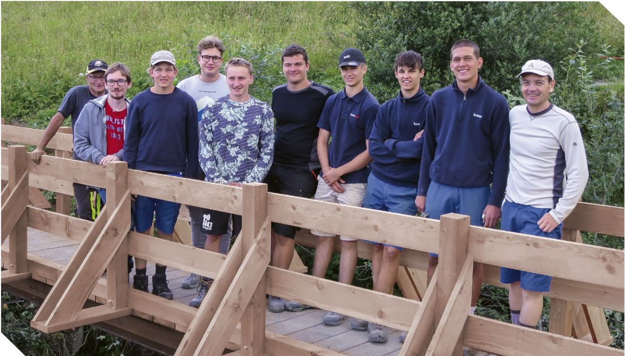
Apprentices from the 2022 Training Camp on the bridge they built themselves in Obersaxen.
