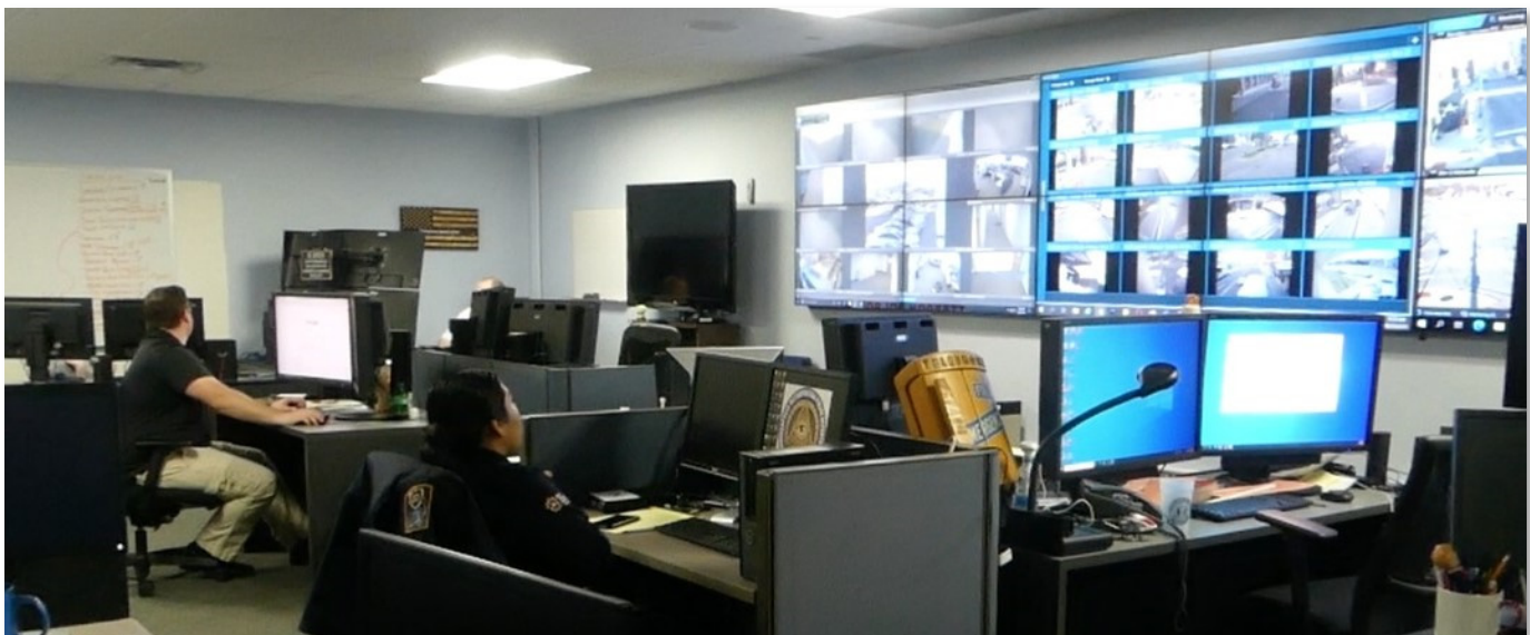
Incident Analysis Center (IAC) personnel monitor a variety of cameras that provide information in real-time. These cameras are located at strategic points all over the city. Some cameras are mounted on mobile platforms that can be moved and set up at designated locations, such as a special event or the scene of a critical incident. This allows command staff to make rapid decisions based upon live video being streamed into the IAC.
