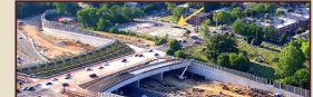
View northwest of the expansion of I-495 in June 2007 bypassing the Centrobanks and Freeman Cemetery (indicated by the yellow arrow). The cemetery would later be restored and it was dedicated as a memorial in 2014. (courtesy)
