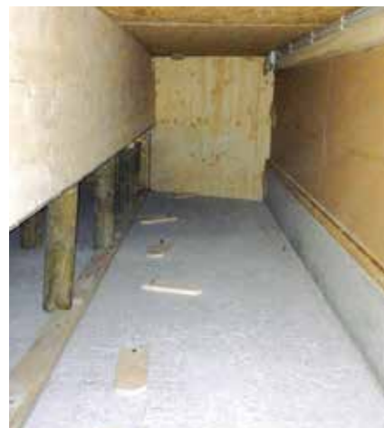
24 Air intake channel
