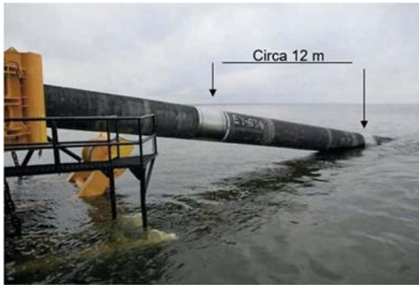
Figure 6: Laying of pontoon pipeline, with detail of the joint between each 12-metre-long module.
