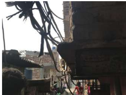
Fig 61 Electrical wires are not proper tied to
