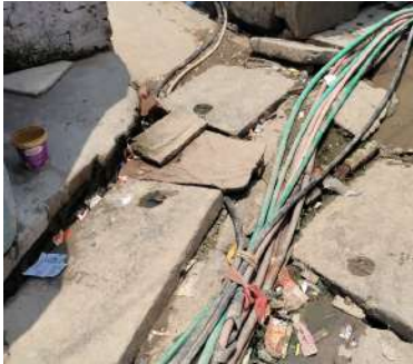
Fig 120 Water connection pipes are laid down on the street openly.
