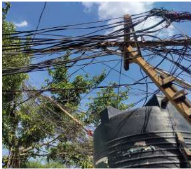
Fig 15 Cluster of wires near the electric poles create unsafe conditions in the Basti.
