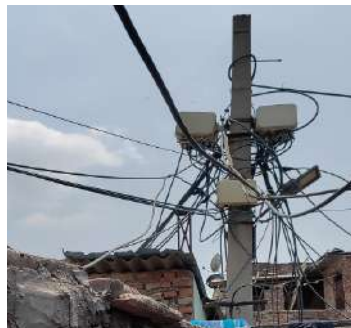
Fig 123 Electricity pole with cluttered wires create unsafe conditions.
