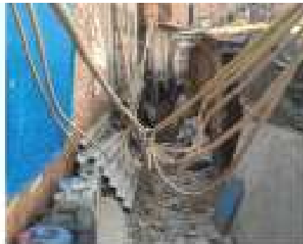
Fig 58 A bundle of electrical cable hung inside Basti,
