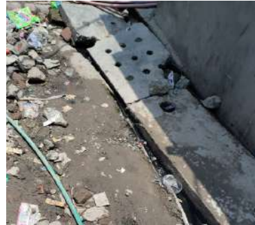
Fig 121 The drains in basti are not covered mostly, if covered are not maintained properly
