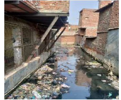
Fig 178 Nullah causing severe hygiene issue as the water overflows during heavy rain.
