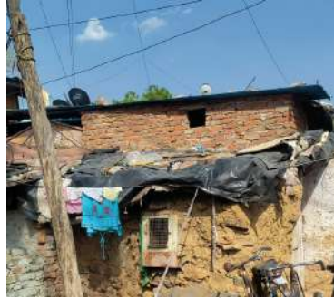
Fig 16 Heat Mitigation through coolers , attached to a mud wall inside the Basti.
