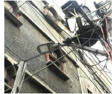
Fig 98 Cluster of Wires in the Basti lead to unsafe conditions.
