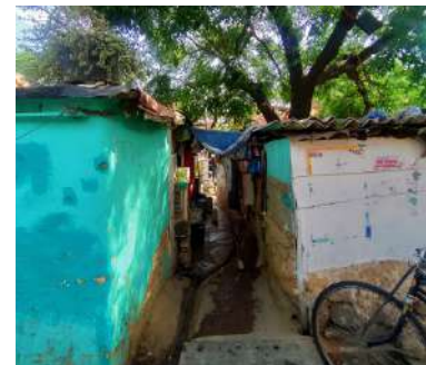
Fig 20 Lack of drainage as per slope leads to water logging on the streets.
