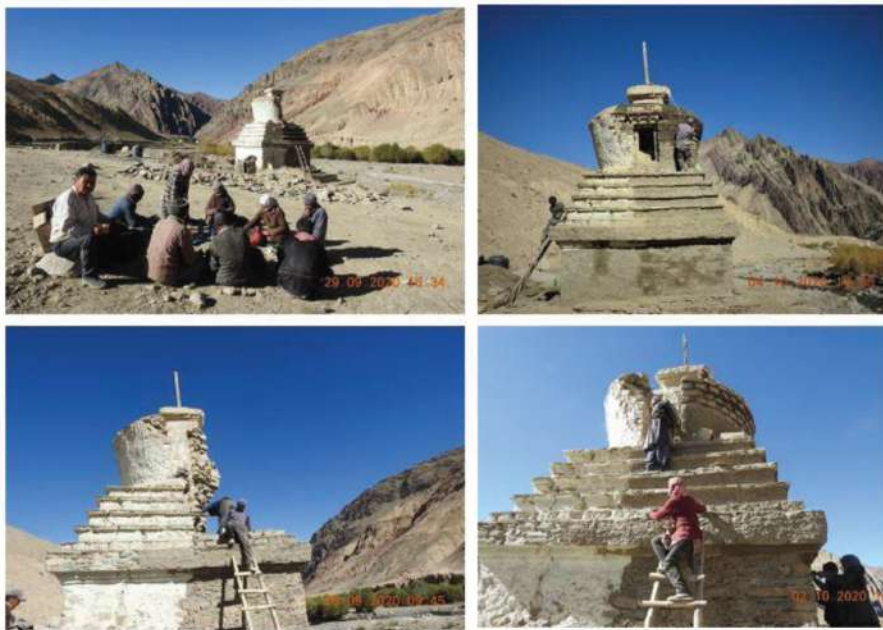
Figure 6: Photos depicting various phases of the conservation work, mud with the straw mixed silty clay mortar plastering holds its joints very strong Source: Karma sonam
